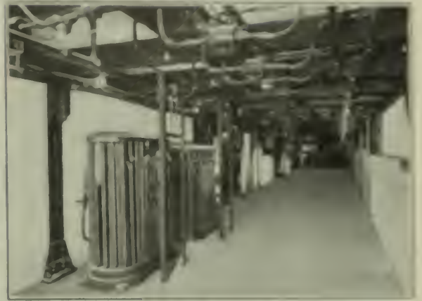
TRANSFORMER GALLERY UNDER SWITCHBOARD
